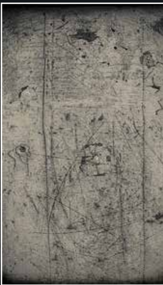
SCRATCHES CONCRETE M L
