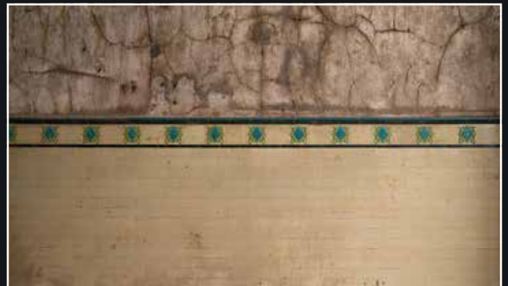
DERELICT TILED WALL
