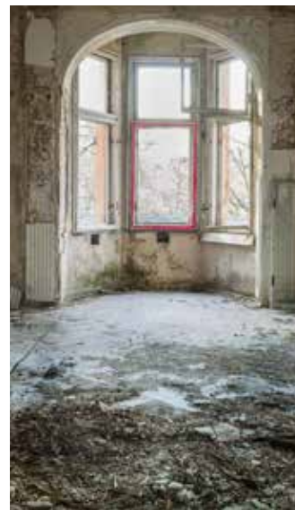
DERELICT BAY WINDOW MMDM
