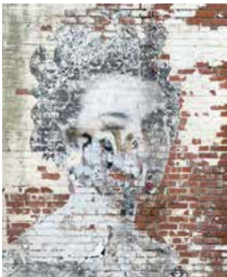
HRH Brick Wall
