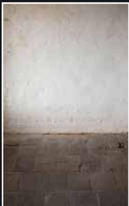
AGED PLASTER WALL FLOOR
