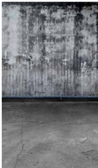
DISTRESSED CONCRETE WALL
