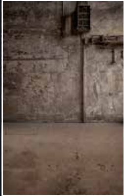
RUN-DOWN FACTORY WALL
