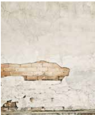
CRUMBLING PLASTER WALL
