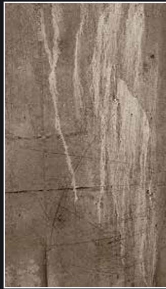
SCRATCHED CONCRETE WALL M L
