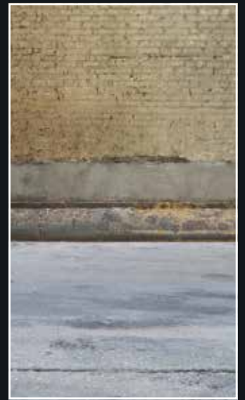
CHICAGO DISTRESSED WALL
