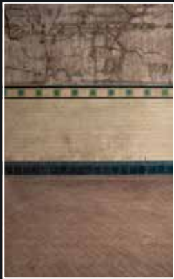
DERELICT TILED WALL
