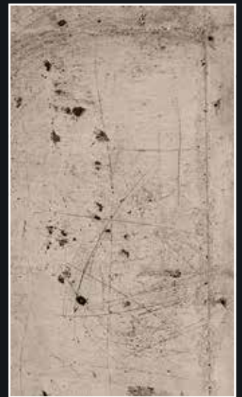
BURNT WALL M L M
