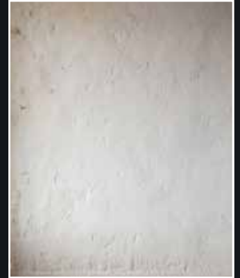
AGED PLASTER WALL
