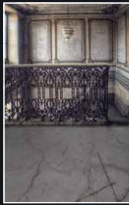
ABANDONED STAIRCASE LD
