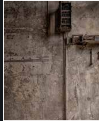
RUN-DOWN FACTORY WALL
